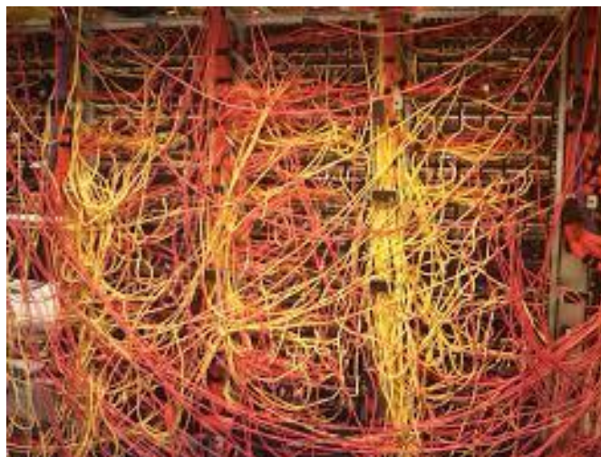
Figure 15 Bad Wiring Closet
